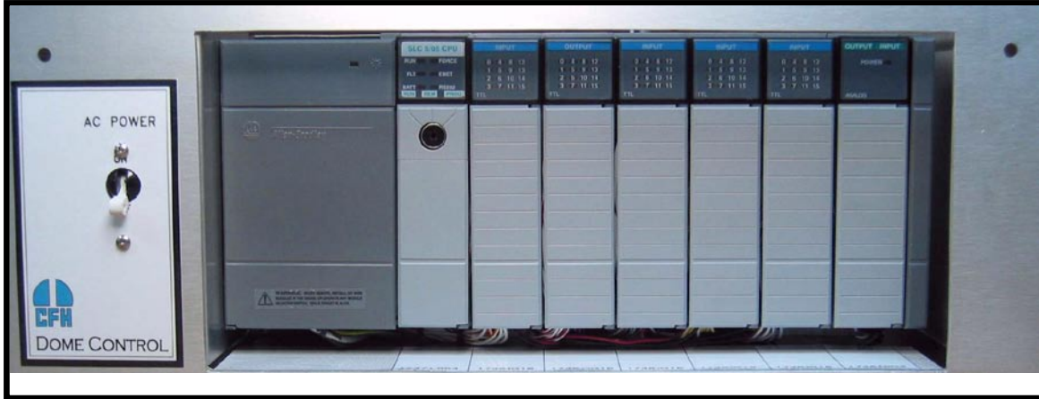
Figure 15: Dome Control PLC in the 4 th floor computer room
