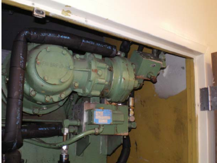
Figure 7: Drive Unit #1 upper door frame
