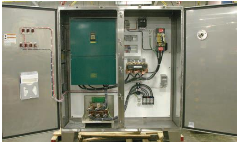
Figure 8: Example motor controller enclosure
